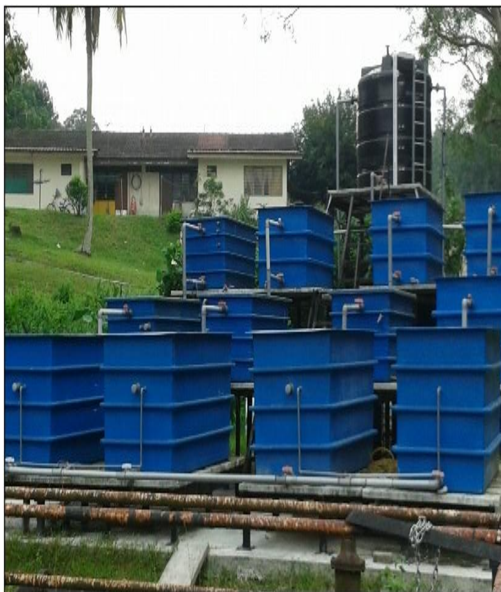
Figure 2. Constructed wetland pilot-scale system in Bukit Putri (UKM)
